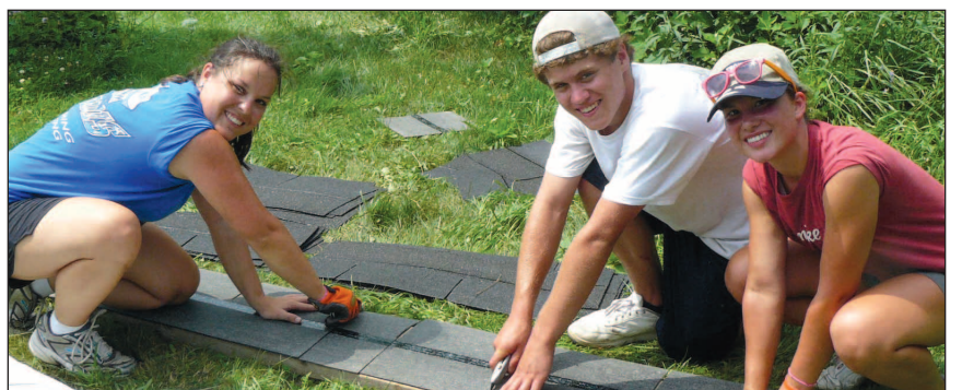
Top photo, Joe Zach, of New York; Scott Springer, of Pennsylvania; Nicki Hayes and Brook LaGreca, also from New York, perch on the rooftop while fixing up a house in Windsor. Above, Kat Spieler, of North Carolina; Scott Lotze, of New York, and Katie Heyl, of North Carolina, cut shingles as part of the Reach Work Camp project that helped refurbish a home in Windsor last week.
